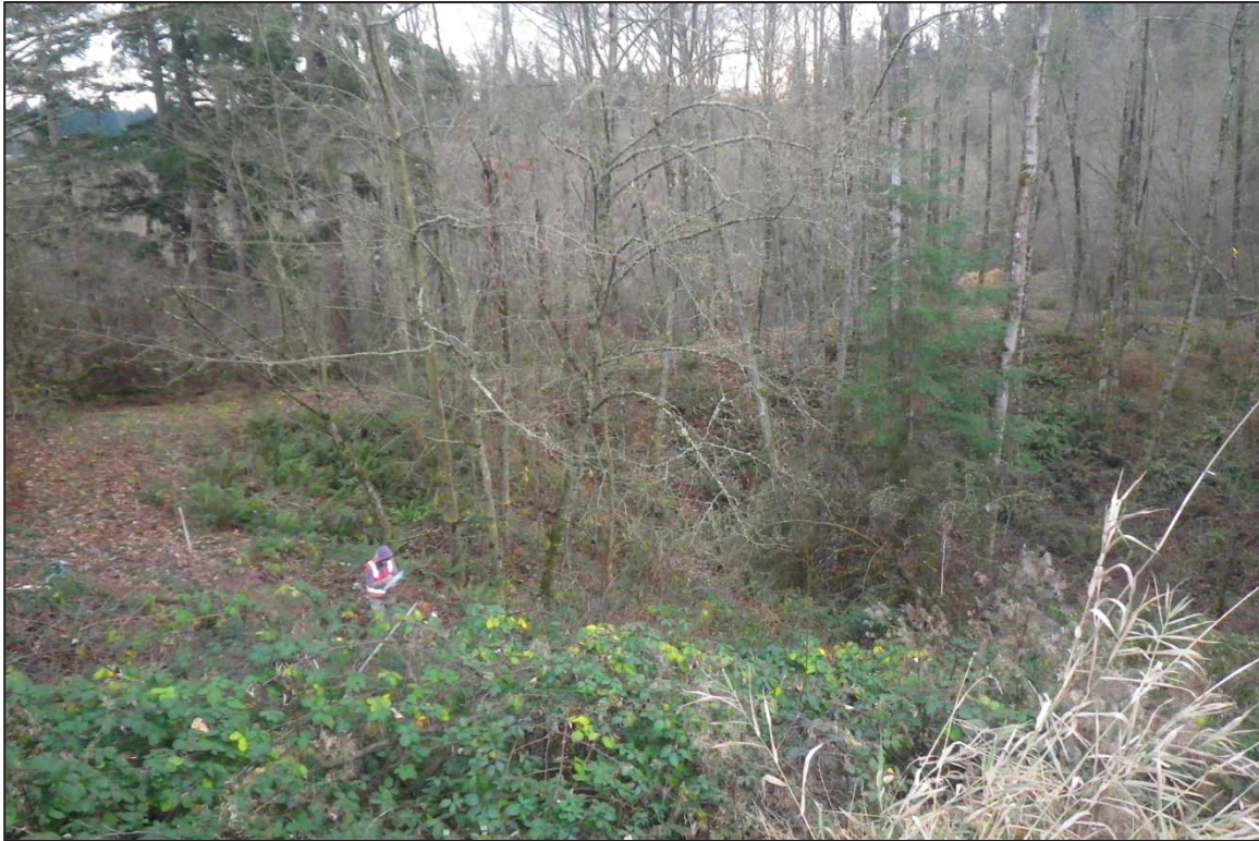
Figure 38. Recently created silt pond between SP 33 and SP 34, showing excavation of SP 33 looking east.
