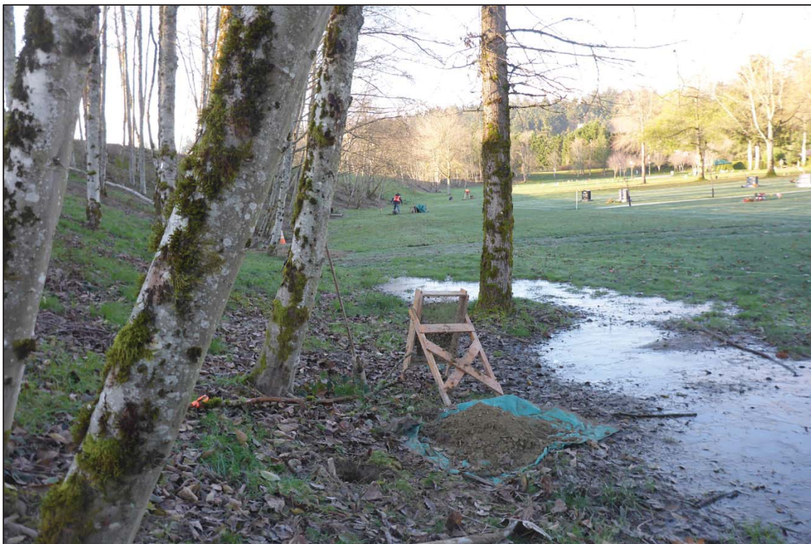
Figure 37. Excavation of SP 32, SP 36, and SP 37 along the base of the artificial berm in the Sediment Pond Area 1b; view to the southwest.
