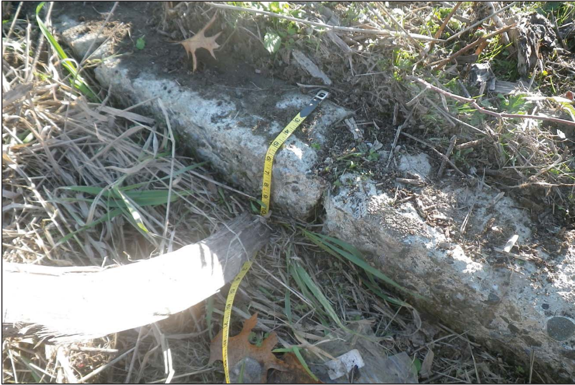
Figure 32. South wall of the foundation feature, which is about 6 inches thick, in 45KI866.
